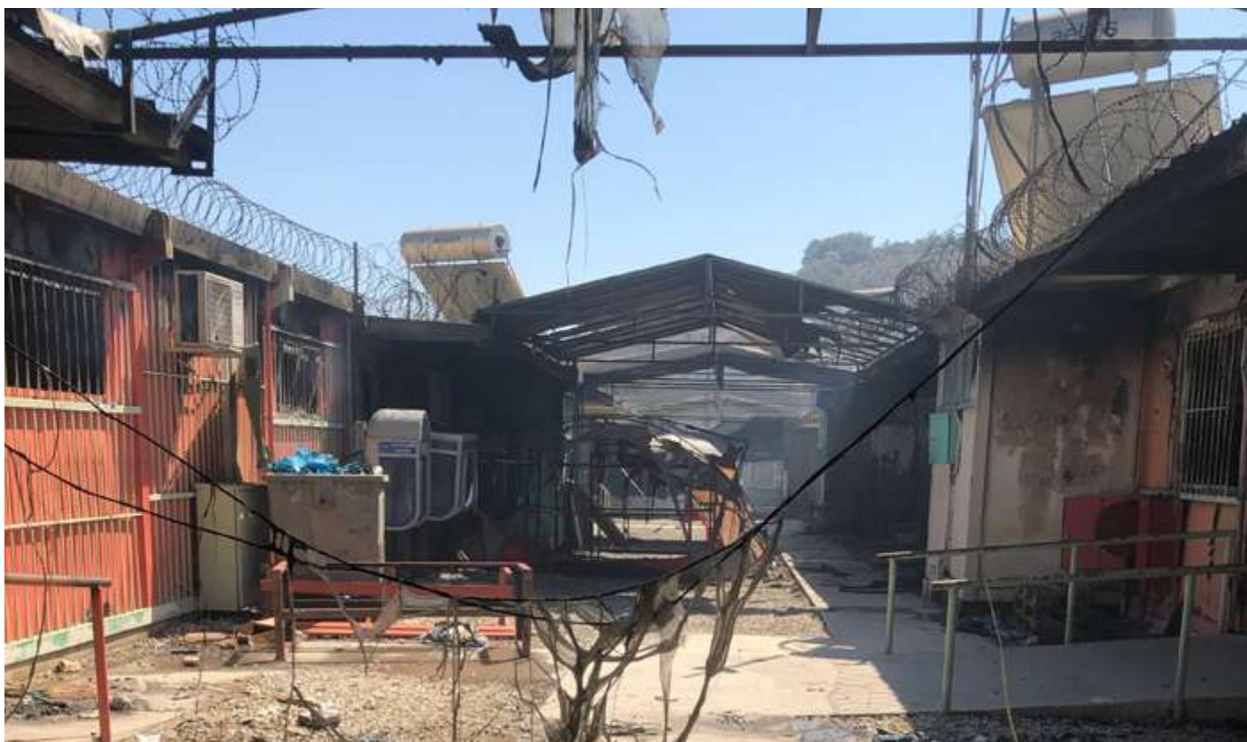
Top: Section A (UASC housing area) was totally destroyed. Photo taken a few hours after the fire.
